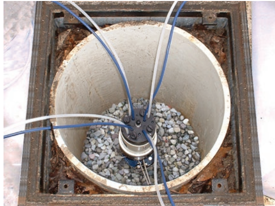
Figure 9-1 Tubing Organized Around the Wellhead
